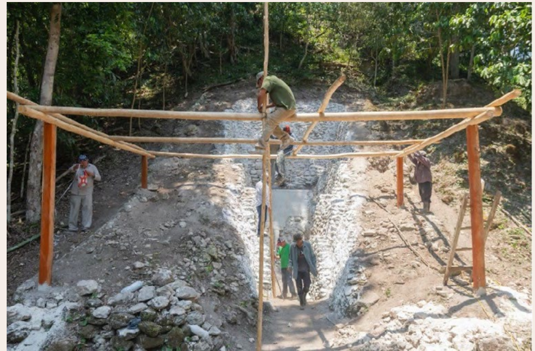
Construction of framework for the preservation of San Bartolo cave murals, Guatemala
