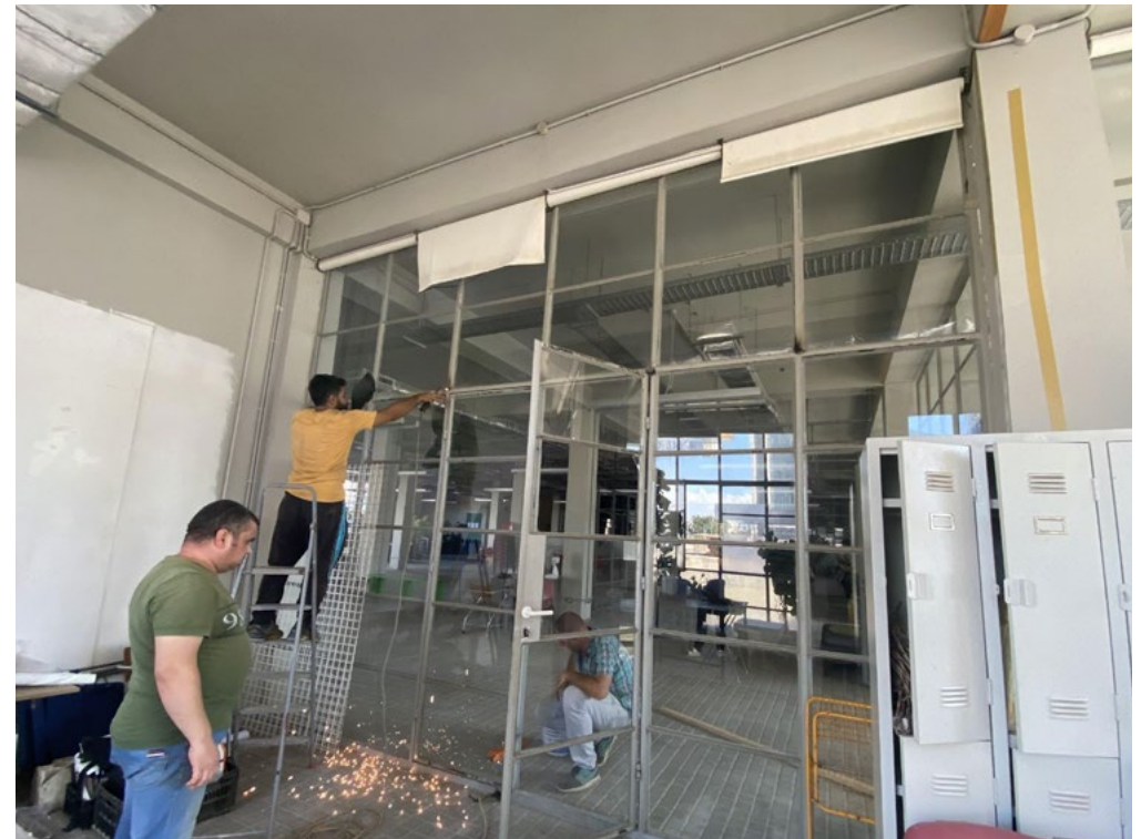
Repairs taking place at the Lebanese Association for Plastic Arts, Ashkal Alwan
