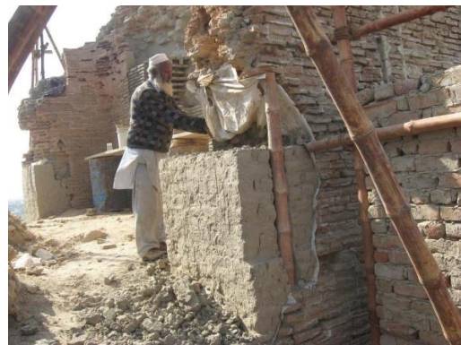
Repairs to a wall using the Heritage Foundation's mud and bamboo technique
