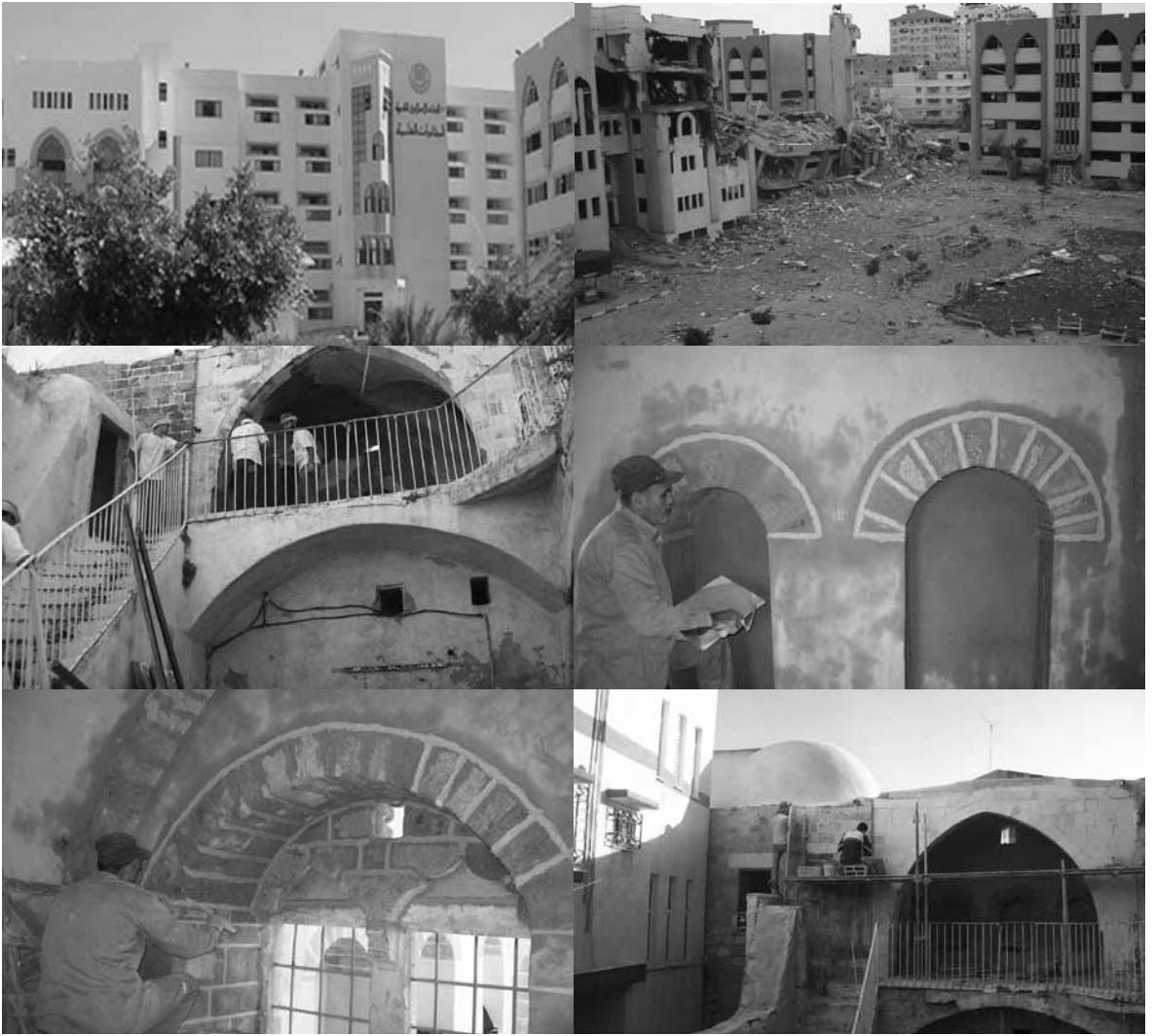
Restoration of the Centre for Architectural Heritage, the Islamic University of Gaza, the Palestinian Territories
