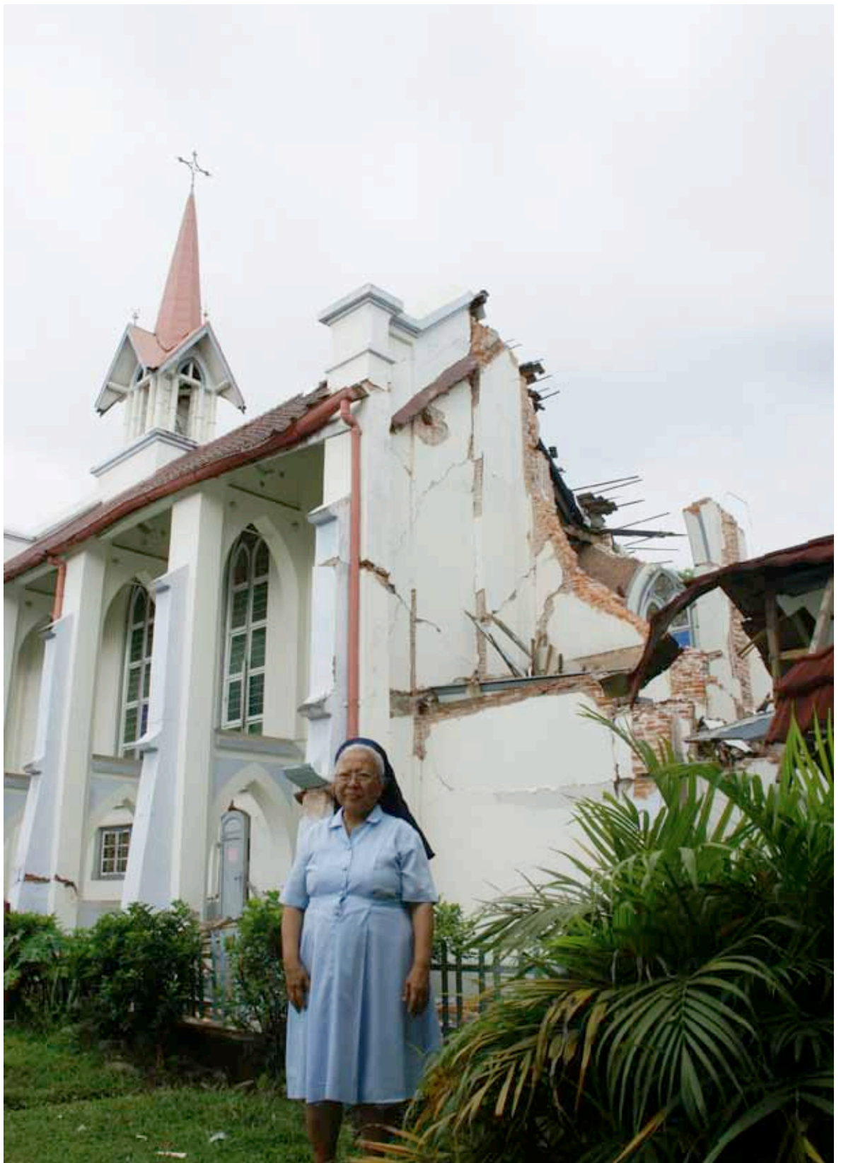
A nun in front of the St. Leo Church on West Sumatra, Indonesia, that was heavily damaged by the earthquake on 30 September 2009
