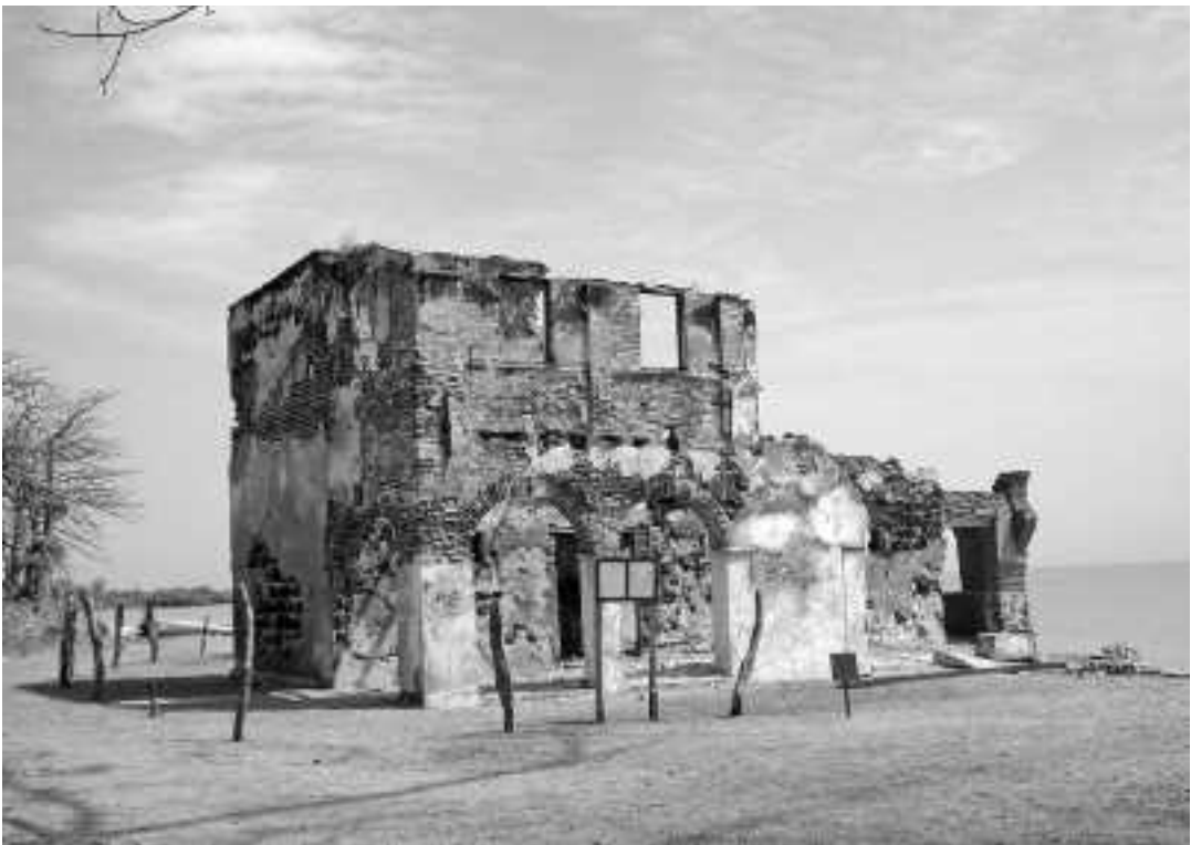
The Compagnie Française d'Afrique Occidentale building in Albreda (Gambia) is being restored with CER's support.
