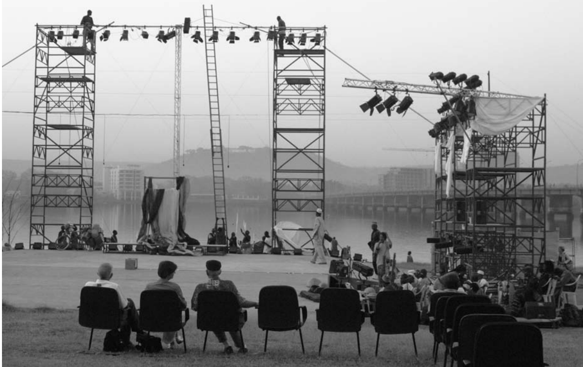
Construction of the stage at the banks of the Niger for the premiere of the Sahel Opera in Bamako, Mali in February 2007.
