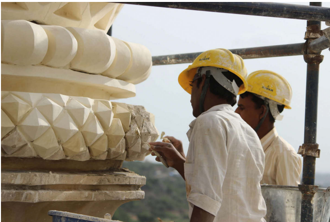
Conservation work (being carried out by the Aga Khan Trust for Culture) on one of the ten monuments supported by the Tata Trusts at the Quli Qutb Shah Heritage Park in Hyderabad, India. Courtesy of Tata Trusts
