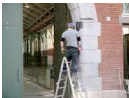
Figure 36 Restoration of De Hallen tram depot in Amsterdam. The project won the Pieter van Vollenhoven Prize of the National Restoration Fund in 2015.
