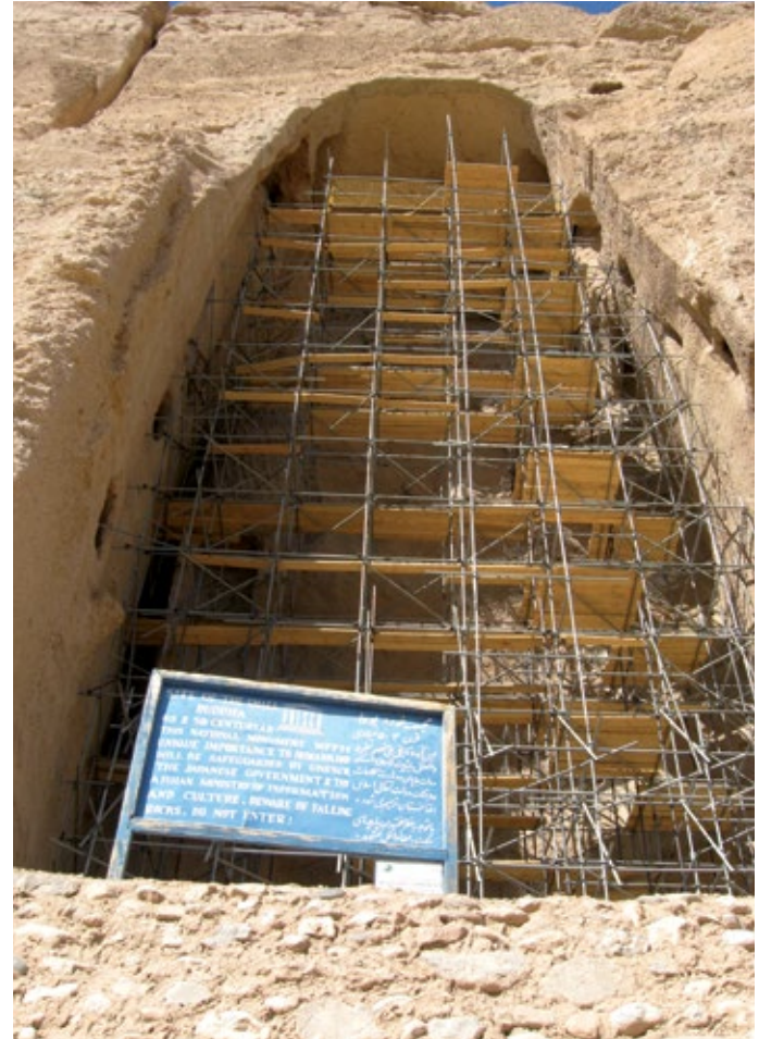
Figure 19. Scaffolding erected to stabilise the crumbling niche of the larger Buddha, at Bamiyan, 2008. Photo by Tracy Hunter from Kabul, Afghanistan (Scaffolding) [CC BY 2.0 via Wikimedia Commons]
